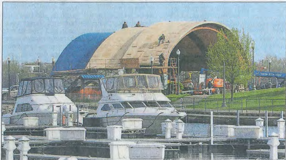
Work crews from Erie's E.E. Austin & Son Inc. install a blue plastic membrane on the roof of the Highmark Amphitheater on Wednesday at Liberty Park. (JACK HANRAHAN/ERIE TIMES-NEWS)
