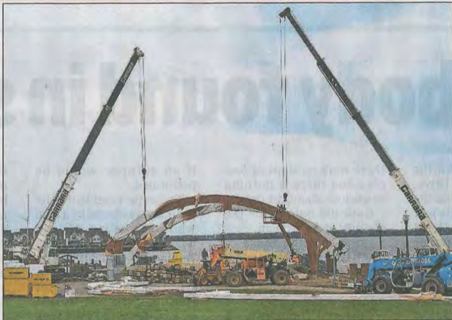
Construction is underway on the new permanent roof at Highmark Amphitheater at Liberty Park on Thursday. Work on the roof is expected to be completed by early May. [DAVE MUNCH/ERIE TIMES-NEWS]
